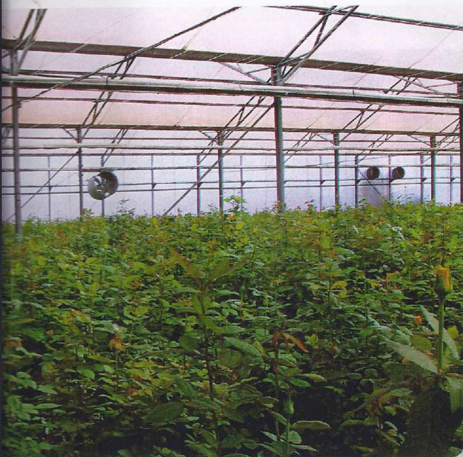
Two Latent Heat Convecter units installed in the greenhouse which measures 30m x 120m. Each unit has two openings which can be seen from the inside. The air is distributed via six circulation blowers.
