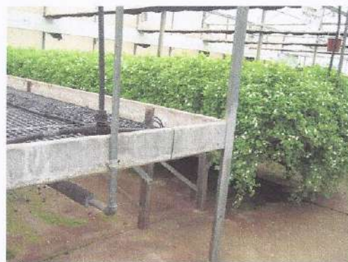
Picture no.5: hot water pipe system under the tables for heat distribution
